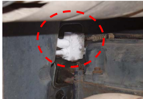
Figure-3. Ice formation layer around the expansion valve.
