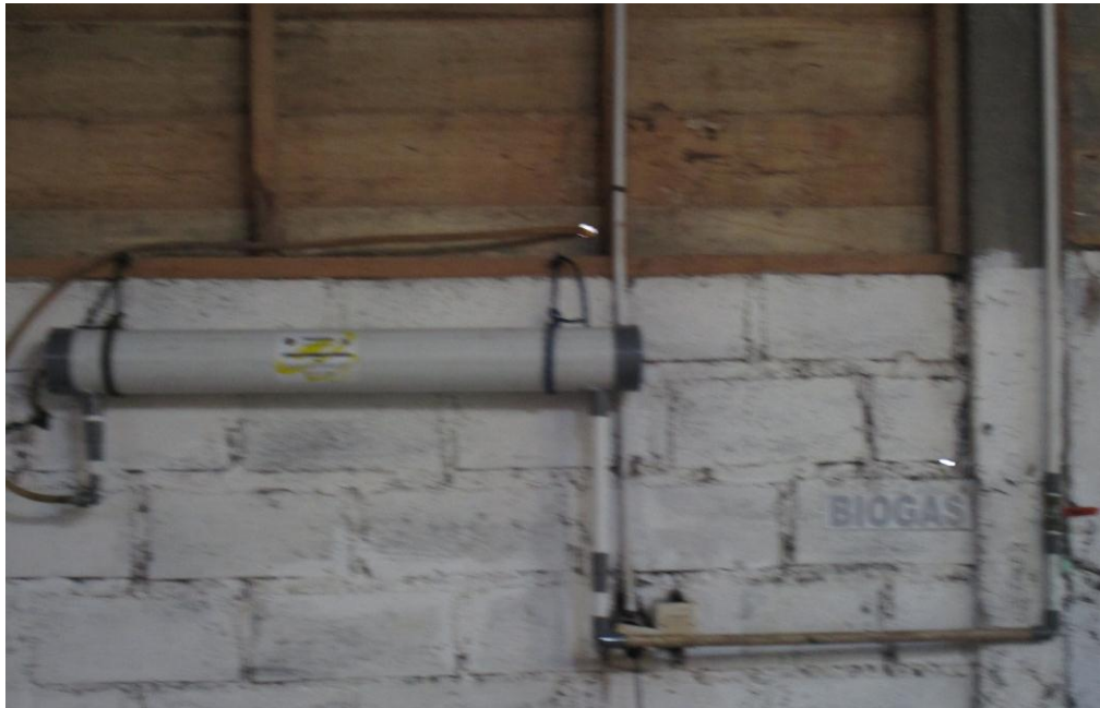
Gambar Instalasi Filter Biogas
